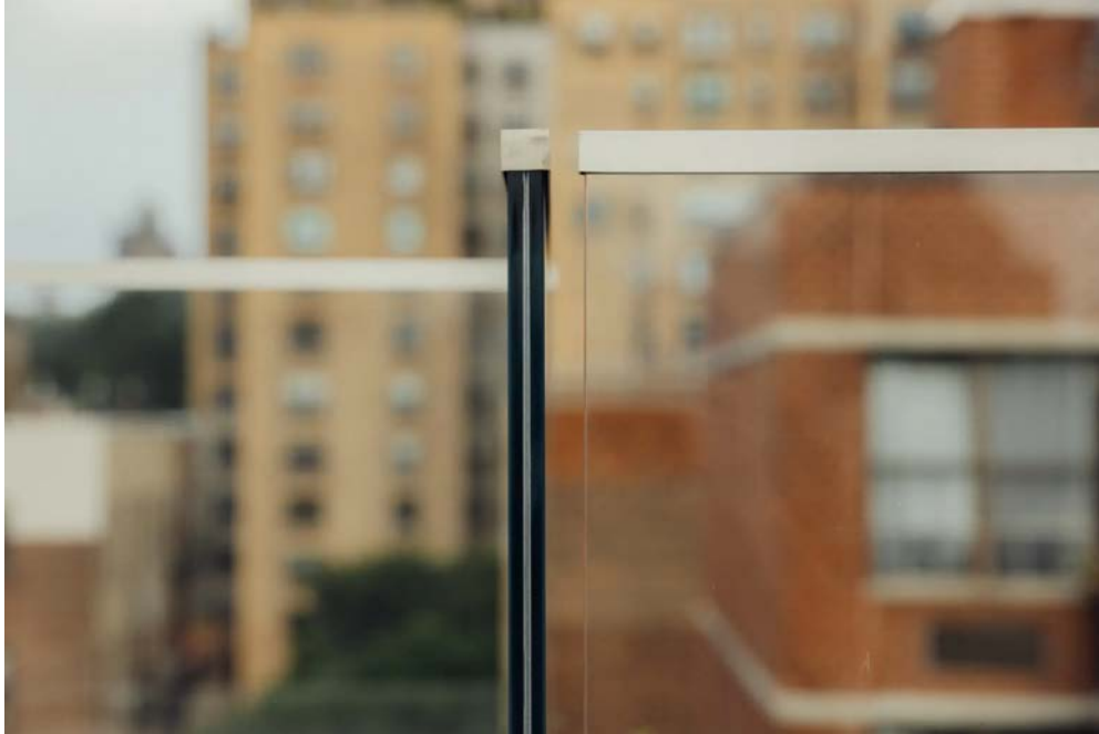
Four panes of triple-glazed glass are used at Charlotte of the Upper West Side. George Etheredge for The New York Times
